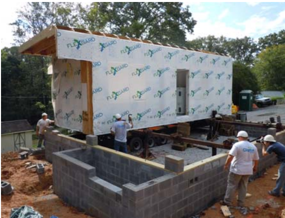
Figure 1: The first modular unit is set onto rollers before being shifted laterally across the staged foundation wall.
