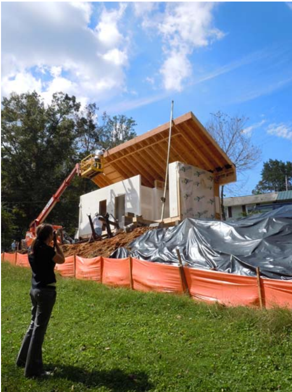
Figure 2: The roof of the first modular unit is hinged into place before temporary supports are installed.
